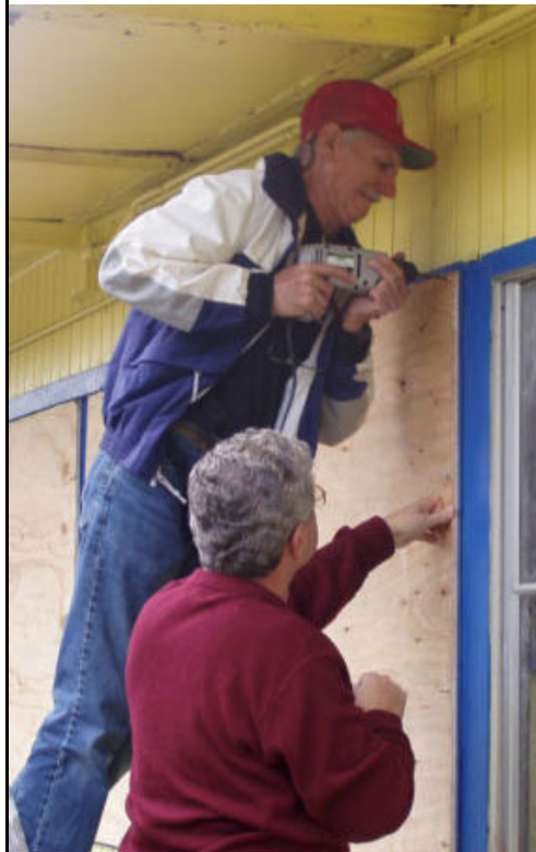
Glen Gray & John Higgins Board up a Window at the Tire Store
