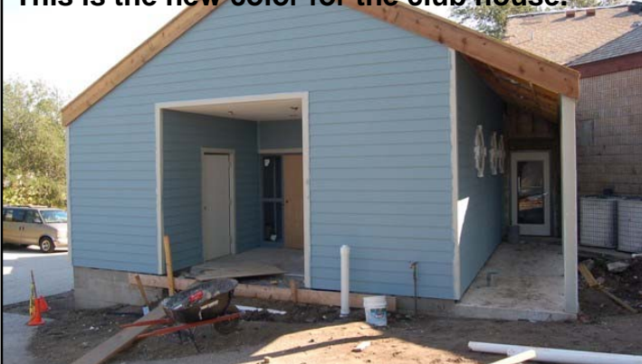
New bathroom and kitchen entrances. This is the new color for the club house.
