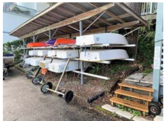
Current Pram Rack in Need of Repair
